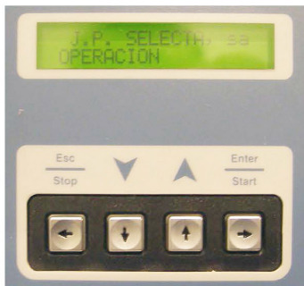
Fig 5.1 Panel de control.
